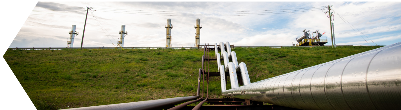
Right: Transport pipelines at Strathcona's Orion asset near Cold Lake, Alta.
